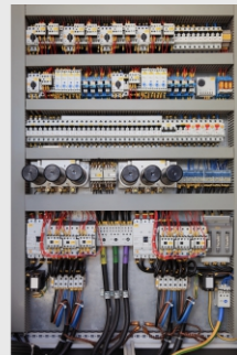
Paneles de control
